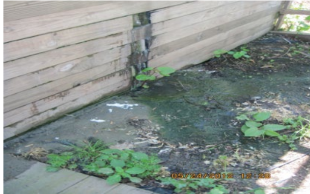
Failed "best fit" replacement septic system in Malletts Bay less than one year after installation.
