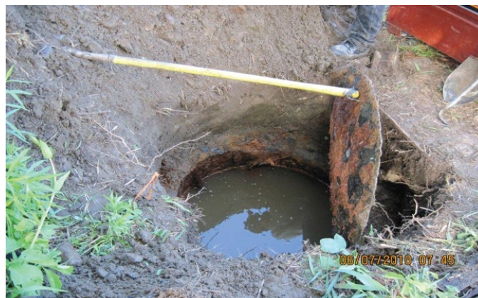
Example of an archaic septic system.
